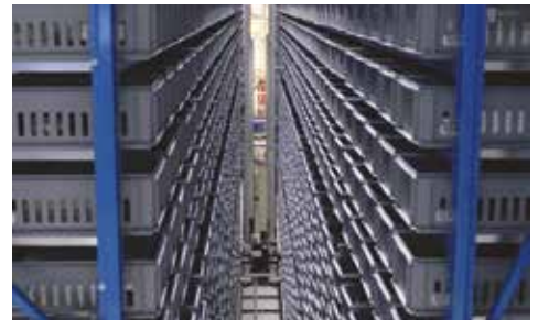
Rail dependent storage and retrieval equipment
